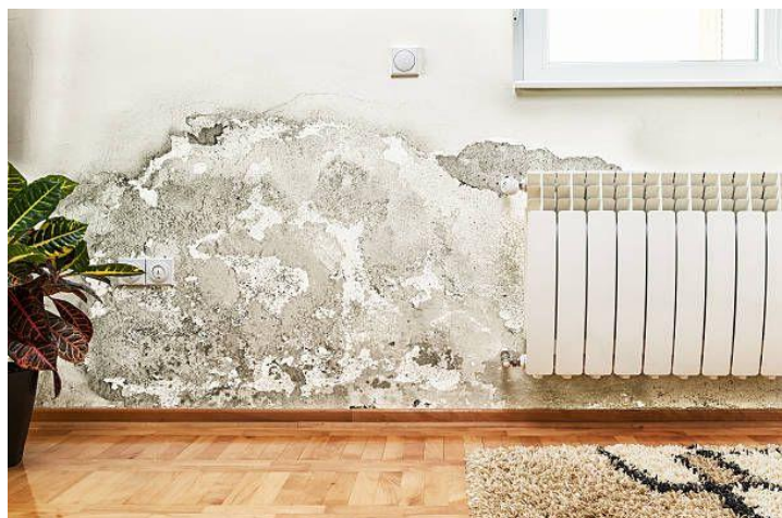
FIGURE 2.EXAMPLE OF DAMPNESS AND MOULD GROWTH ON INTERIOR WALLS
