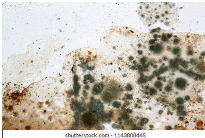
Figure 3: Excess mould on the wall.
